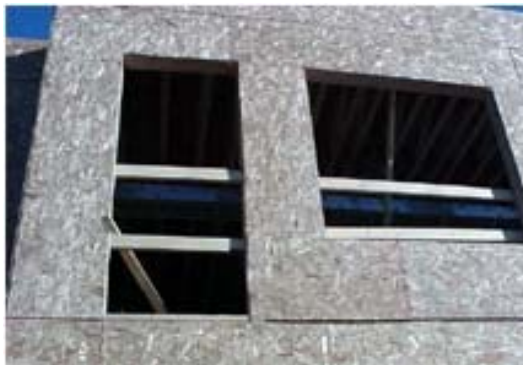
Figure 35 - Guardrails protecting window openings.
