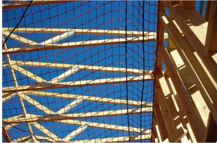
Figure 7 - An example of a safety net system.
